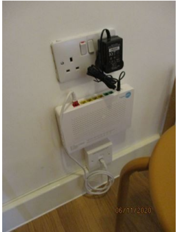
Image 12: HALLWAY Modem to wall
