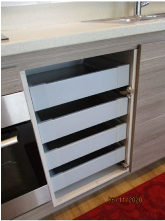
Image 35: LIVING ROOM AND KITCHEN door broken off
