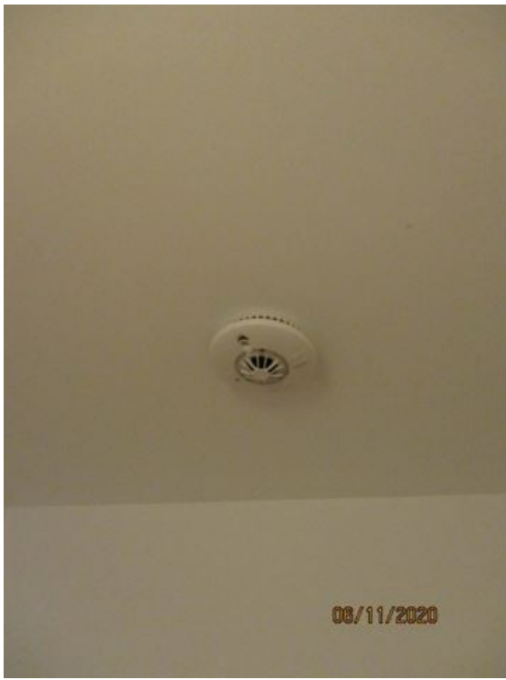
Image 9: HALLWAY additional fire alarm
